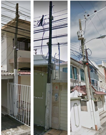
Figure 1. Utility poles close to buildings (houses).
